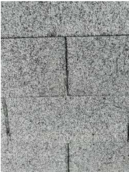
Granular loss noted on shingles edges
