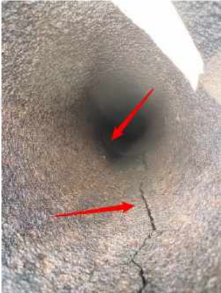
crack extends down below the roof line
