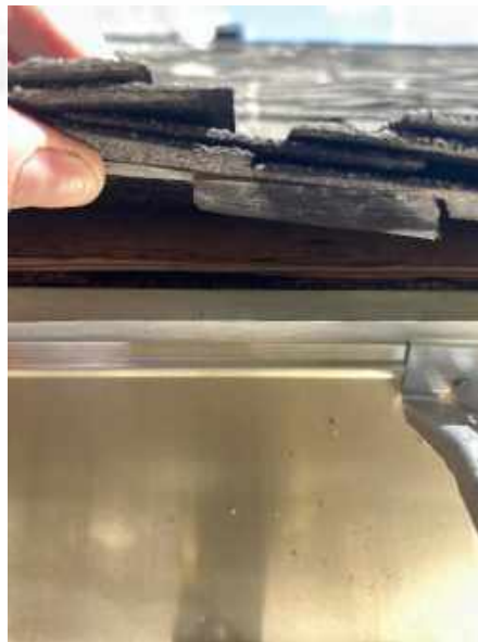
Missing drip edge and waterproofing underlayment on the upper rear roof section.
