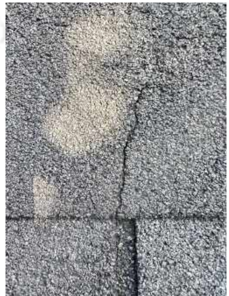
surface cracking lower rear roof
