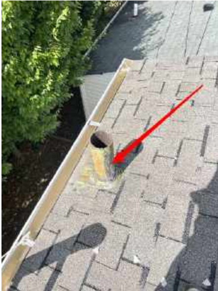
cracks visible on exterior of pipe
